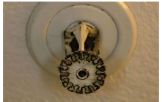
Corroded sprinkler head
